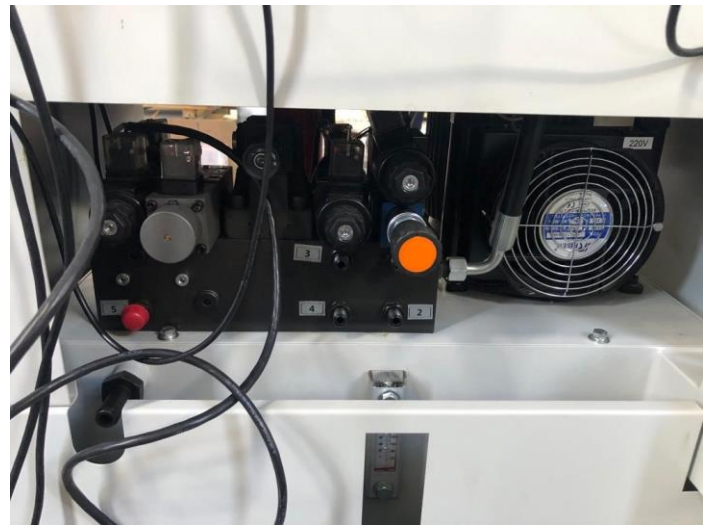
Back view of the controller
